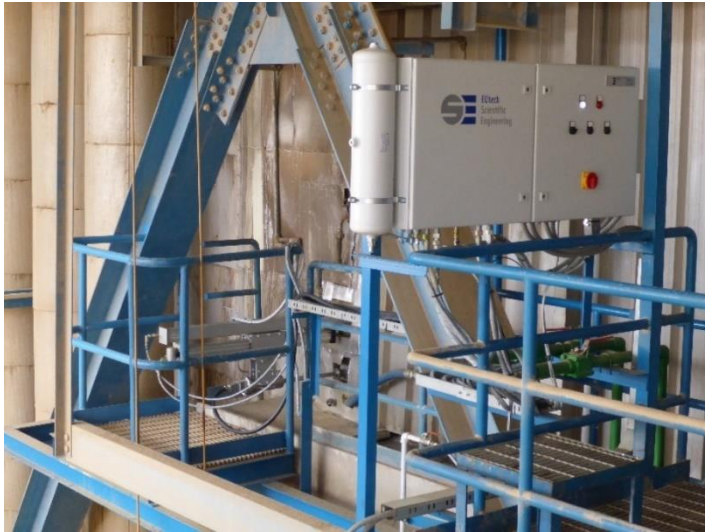
Figure 5: EUvis - control and retraction units (left boiler wall)
