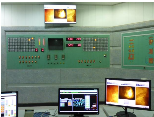
Figure 6: Online visualization in control room
